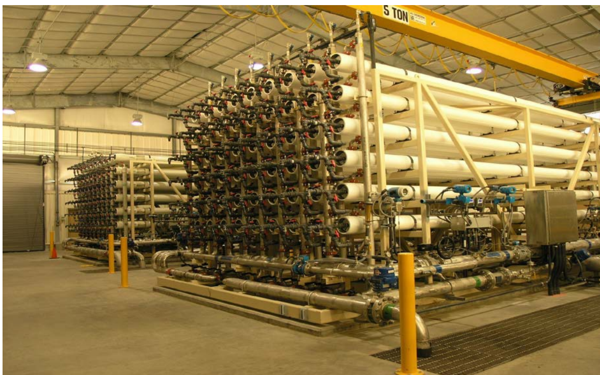
Figure 2-2. The Bingham Canyon Water Treatment Plant RO skids. Each white vessel contains seven spiral-wound membrane units. Photo courtesy of Kennecott Utah Copper, LLC.
