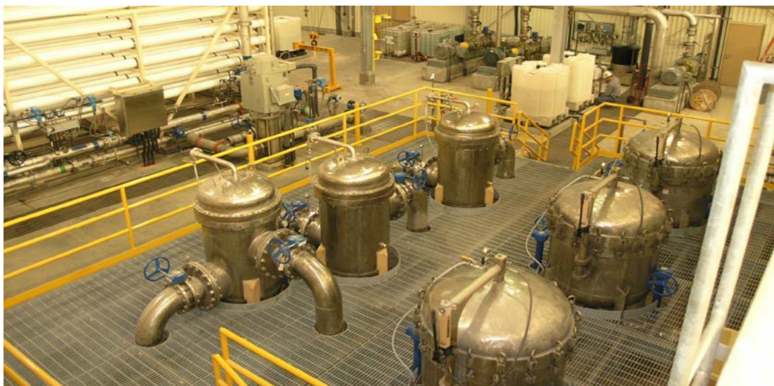
Figure 4-1. Kennecott's BCTWP bag and cartridge pretreatment equipment. Photo courtesy of Kennecott Utah Copper, LLC.
